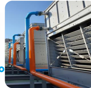
Cooling Tower / Circulating Water Pump
